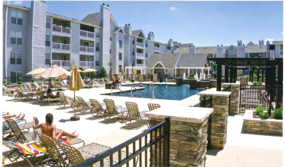
Klæ Construction had to hoist the building materials over the four-story structures during the renovation of the four interior courtyards for Mountain View Crossing in Wayne, N.J.
